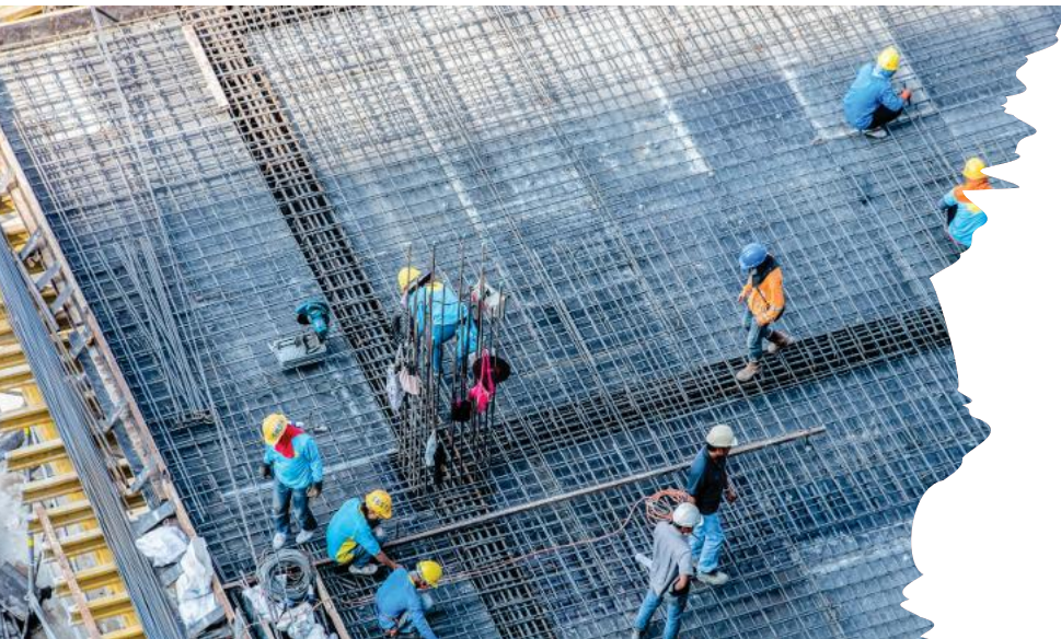
Earthquake-resistant construction is rarely incorporated into building projects due to lax regulations
