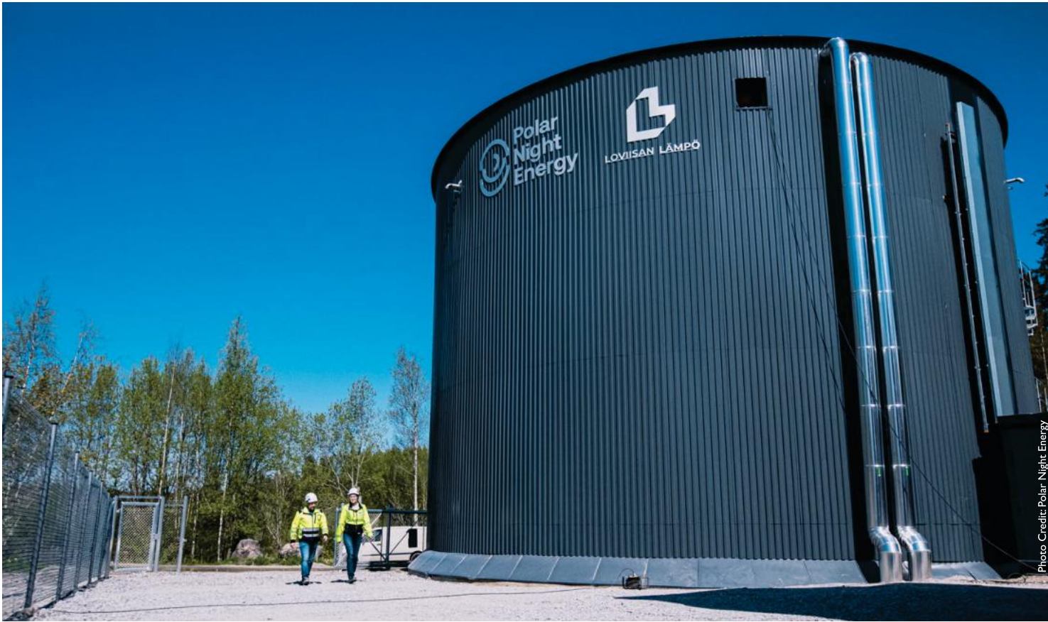
The Polar Night ‘sand battery’ in Pornainen, Finland, can cover almost a month of the small town’s heating demands in summer and nearly a week’s in winter, cutting oil use by storing energy as heat.
